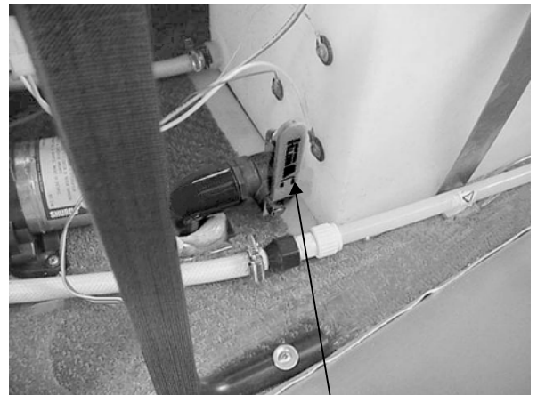
Water Tank Drain Valve
