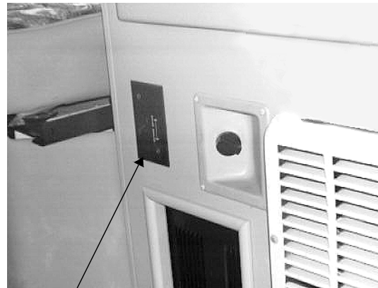
Water Heater Power Switch
