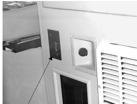
Water Heater Power Switch
