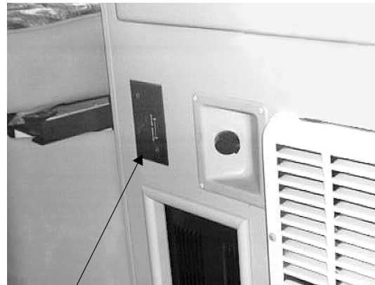
Water Heater Power Switch
