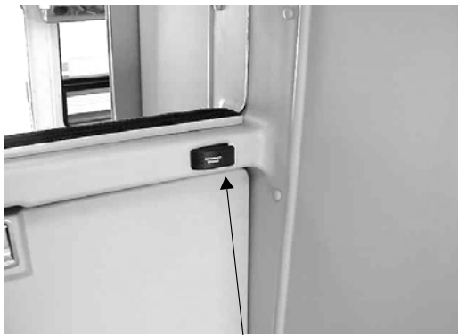
Shower Drain Pump Switch
