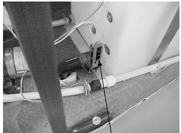
Water Tank Drain Valve
