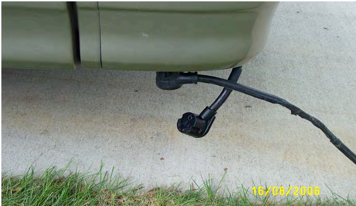
Female 30 Amp plug [that has been fitted to the vehicle end of the severed original shore line cable], attached to the mounted 30 Amp Male plug [not visible]. The 30 Amp cord and Female plug from the generator are hanging down, waiting to be attached when you will leave camp, or for dry camping.
