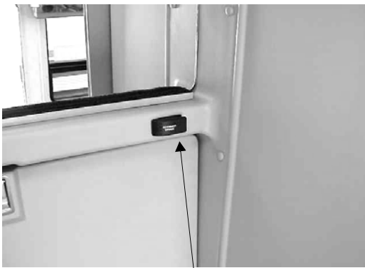
Shower Drain Pump Switch
