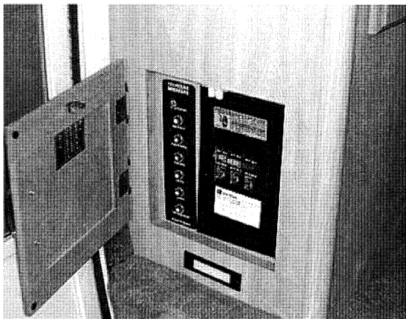
12-Volt Breaker Panel - Model 22FD
