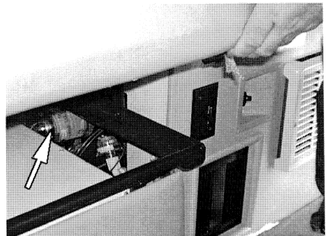
Model 22FD: The shower pump is located below an access hole beneath the bedboard at the foot of the rear bed in the left (driver side) rear of the coach.
